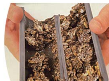
Pipe clogged with zebra mussels
